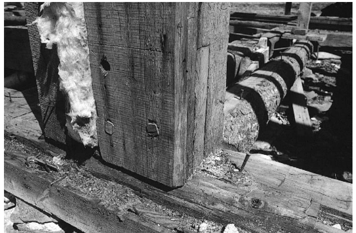
A free tenon in the bottom of a post in this house in Windsor, Mass., may be a repair or a fix for a mistake. Shadows are cast by joists above.
