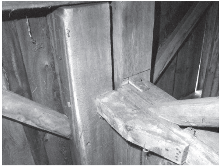
When the builder added to this barn in Savoy, Mass., he saved on a new 30-ft. tie beam by framing a piece into the post and pinning and nailing it to the existing barn's tie beam. Sheathing remains in place below tie beam; shallow wedge for dovetail tenon emerges on surface.
