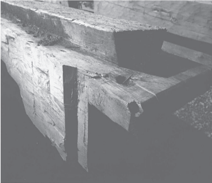
Sixty-ft. 14x17 hemlock sill girder from a barn in Middleburg, N.Y., rabbeted and undercut on both sides for 3-in. threshing-floor planks. Girder was blind-tenoned to gable sill and secured by three pins.
