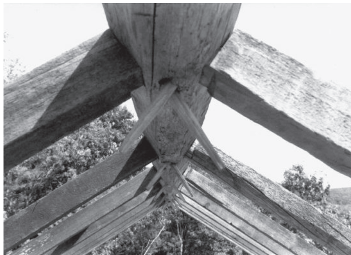
View down the ridge beam of a mid-19th-century 40x50 barn in Hinsdale, Massachusetts. The 3x4 rafters have barefaced tenons.
