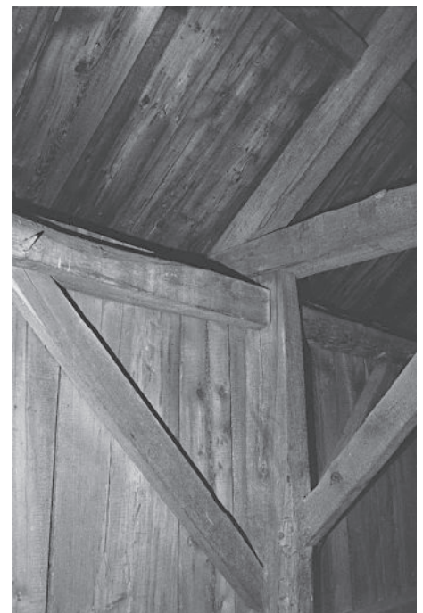
English tying joint tradition lives on after a fashion, with dropped, interrupted plates, in this Newfields, Maine, aisled barn. The plates tenon into the sides of the post; a flying plate (not visible) is supported by the tie beam ends.
